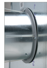
Sheet Metal Trunkline
