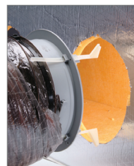
Duct Board Trunkline
